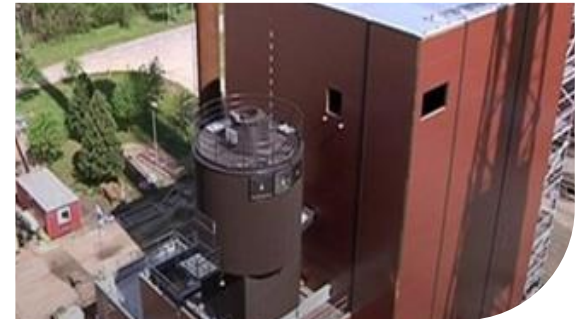
First demonstration scale integrated pyrolysis unit, Fortum
